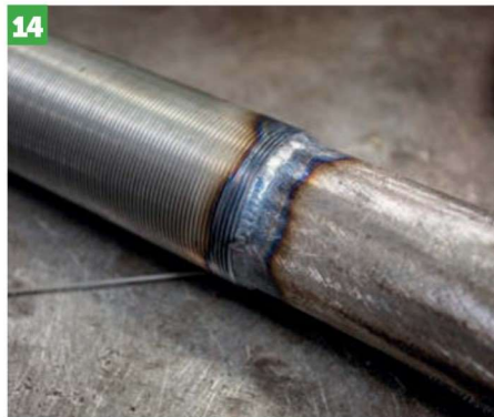
You want a continuous run of weld all the way round. Once happy, clean up the welds if necessary. Now's also a good time to add a lick of paint to the strut body.
