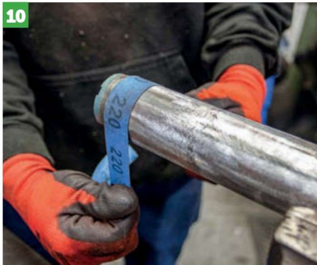
The final job prior to welding the sleeve in place is to clean up the metal near the top of the tube by hand using emery paper.
